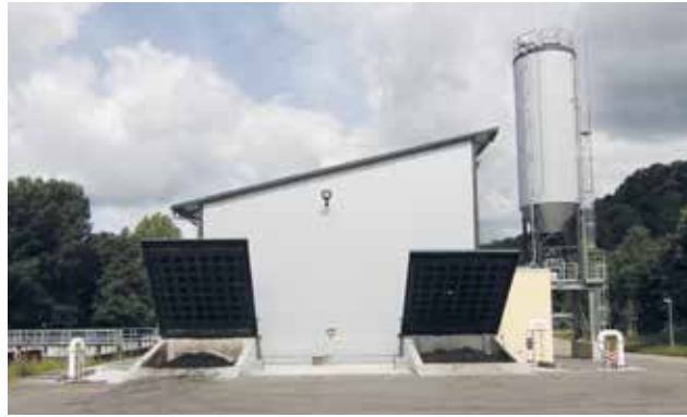
Sludge bunker and dry material silo.
