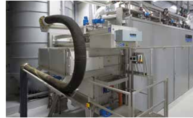
Sludge feeding with HUBER extruder unit.
