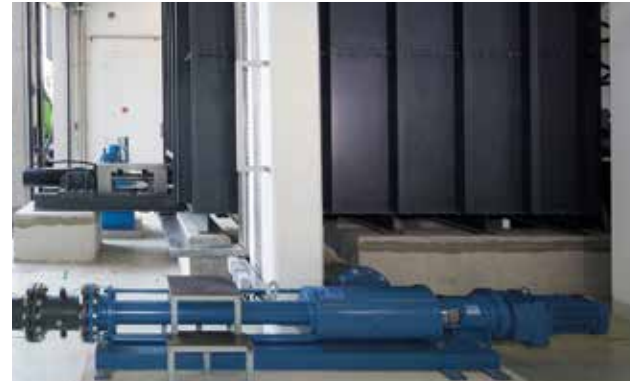
Sludge bunker and pump.
