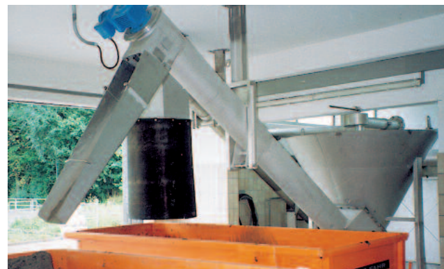
A classifying screw transports the grit from the separation room into a skip.
