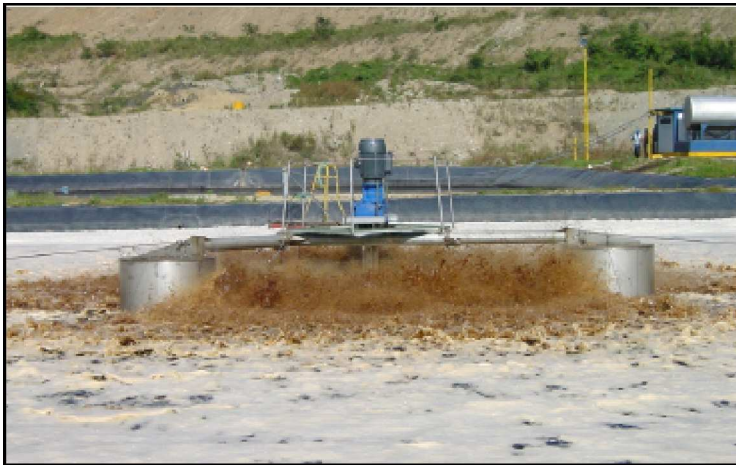
Typical TWISTER™ Low Speed Aerator on floats.
