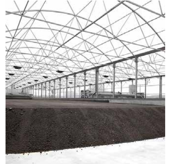
Dry sludge for removal by wheel loader and truck.
