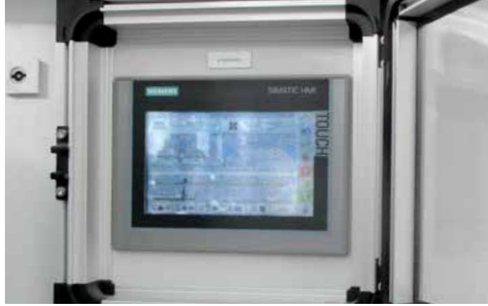
Touch panel for plant control.
