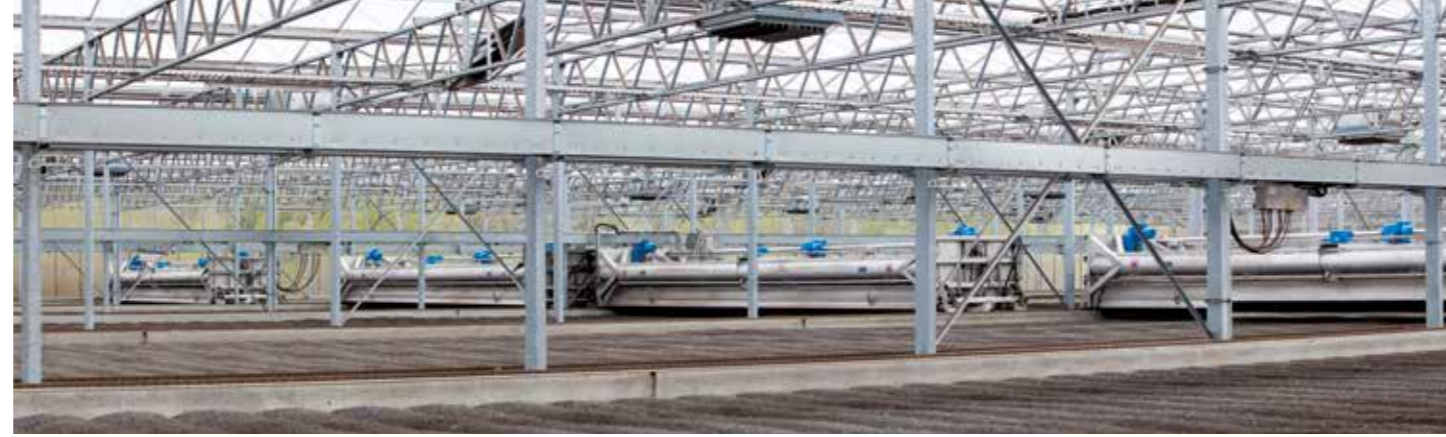
Parallel operation of HUBER Sludge Turner SOLSTICE® units.
